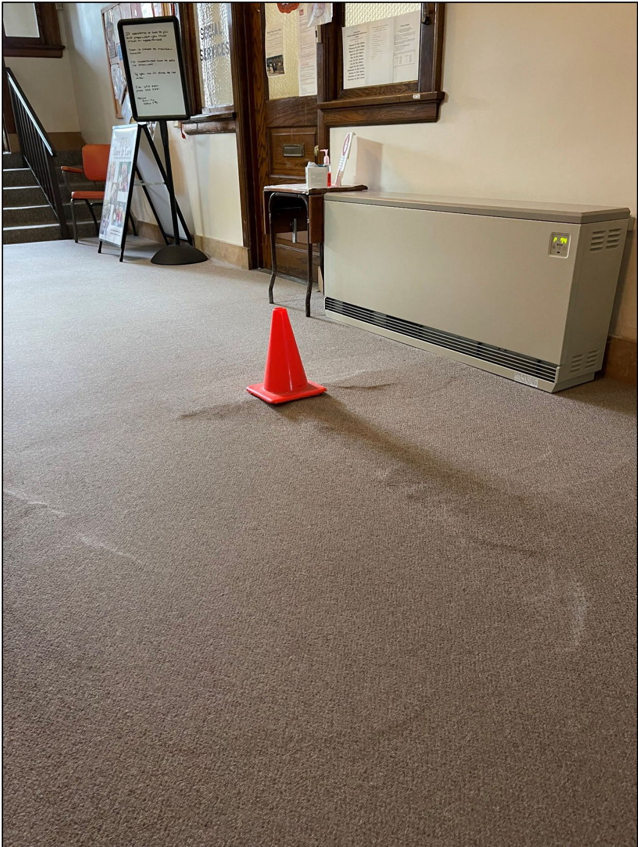
Figure 6.4 – Foster County Courthouse Substructure Heaving #2
