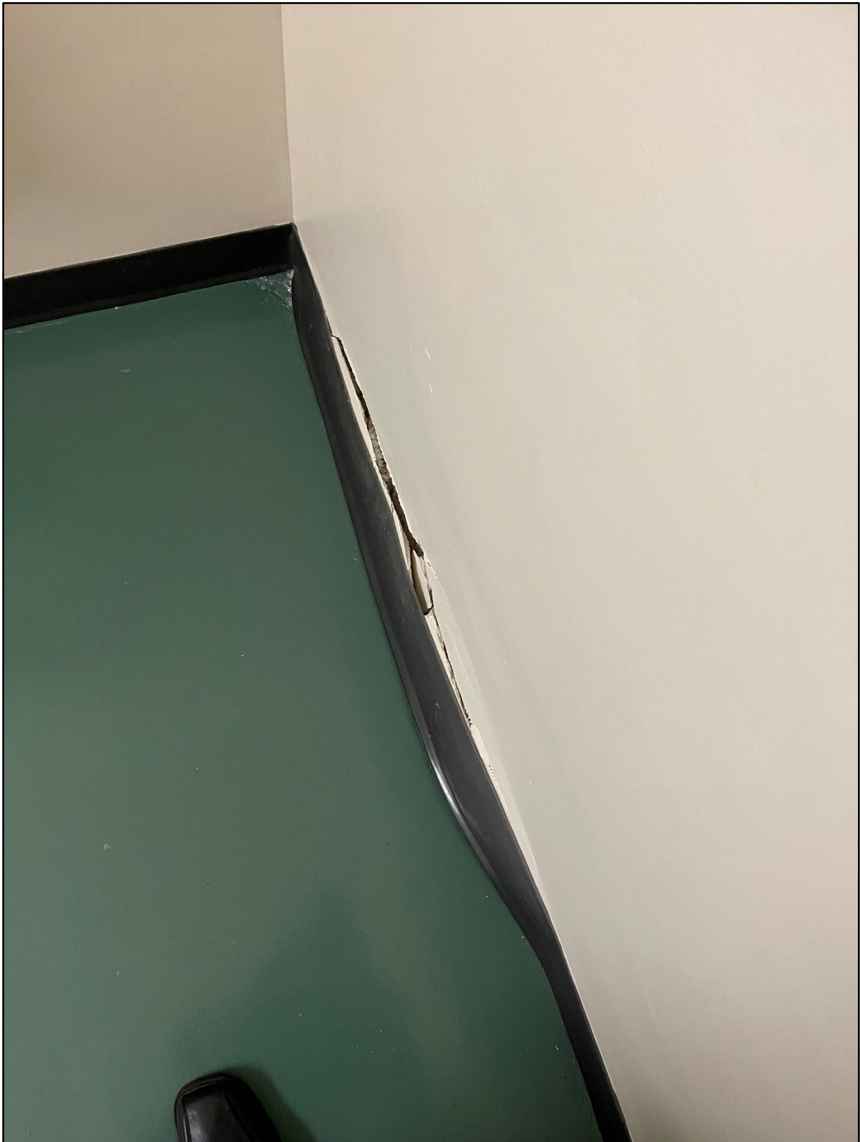
Figure 6.5 – Foster County Courthouse Substructure Heaving #3
