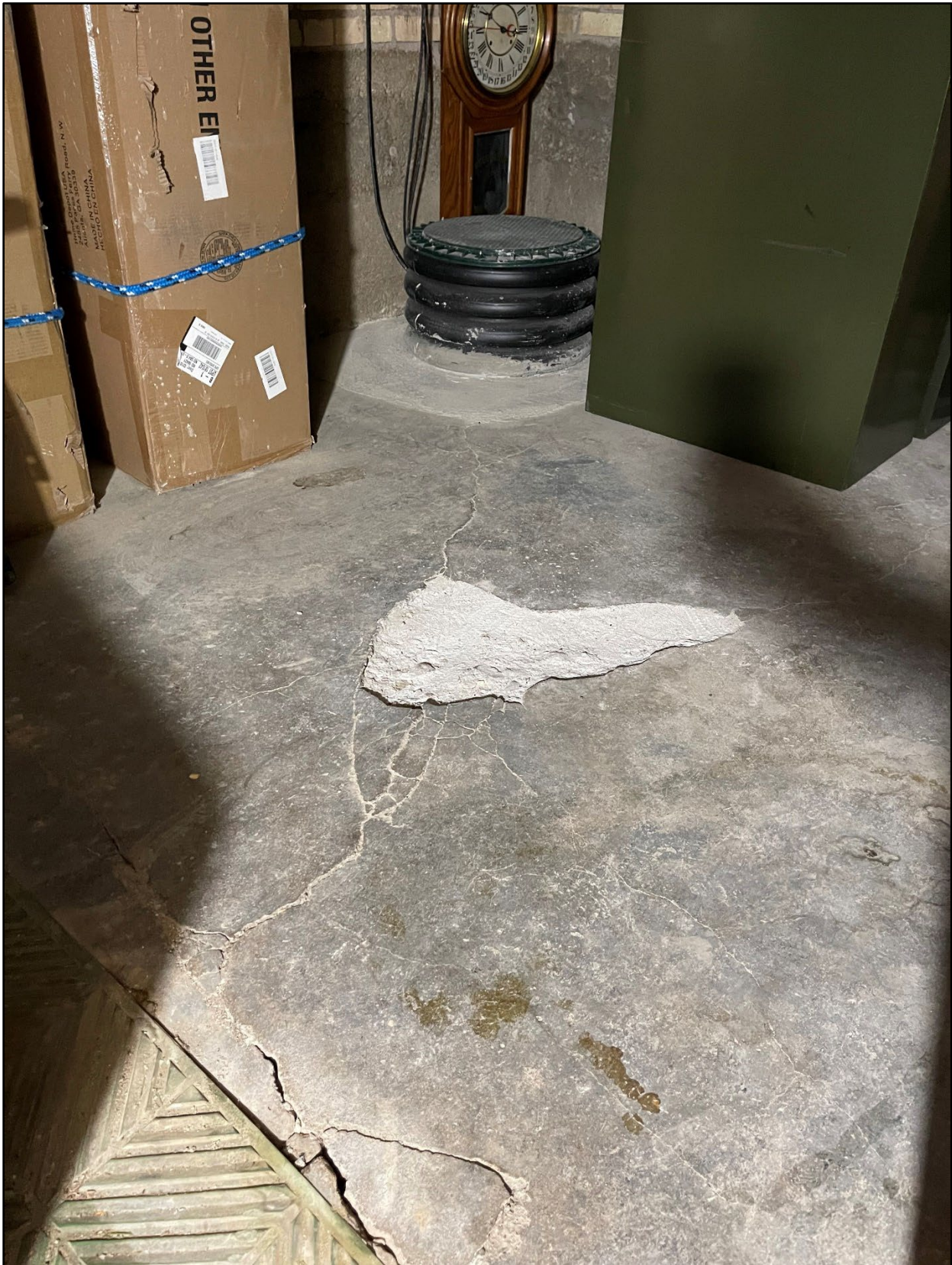
Figure 6.3 – Foster County Courthouse Substructure Heaving #1
